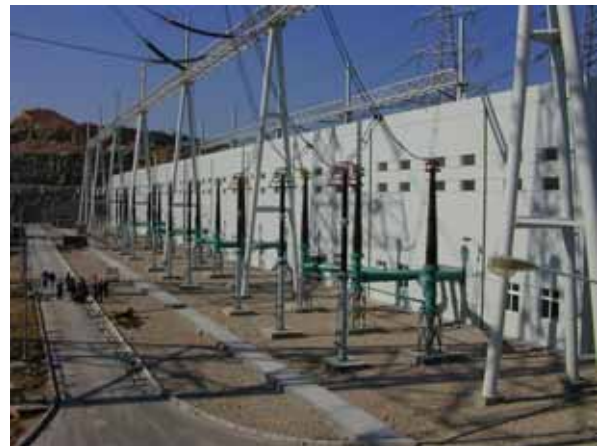
In a 550kV system (1997)
