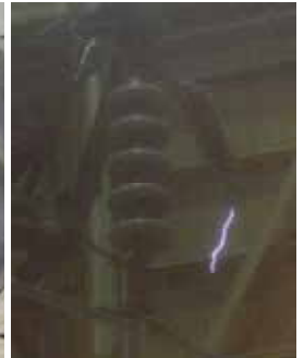
Insulation Coordination Test
